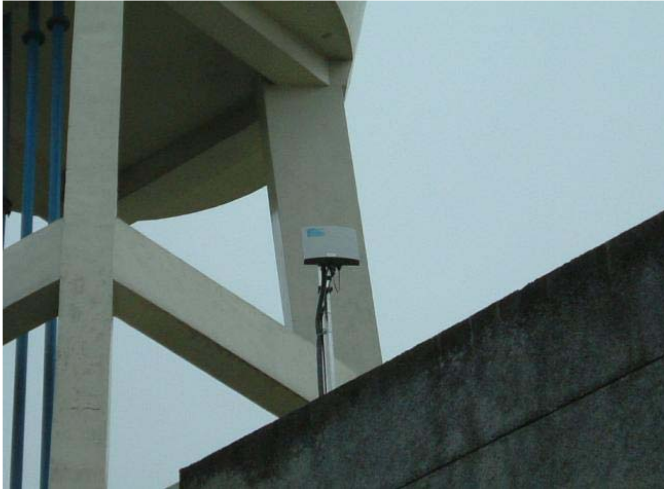
WL-2401 (flat panel antenna integrated) On roof of Veteran Care Center
