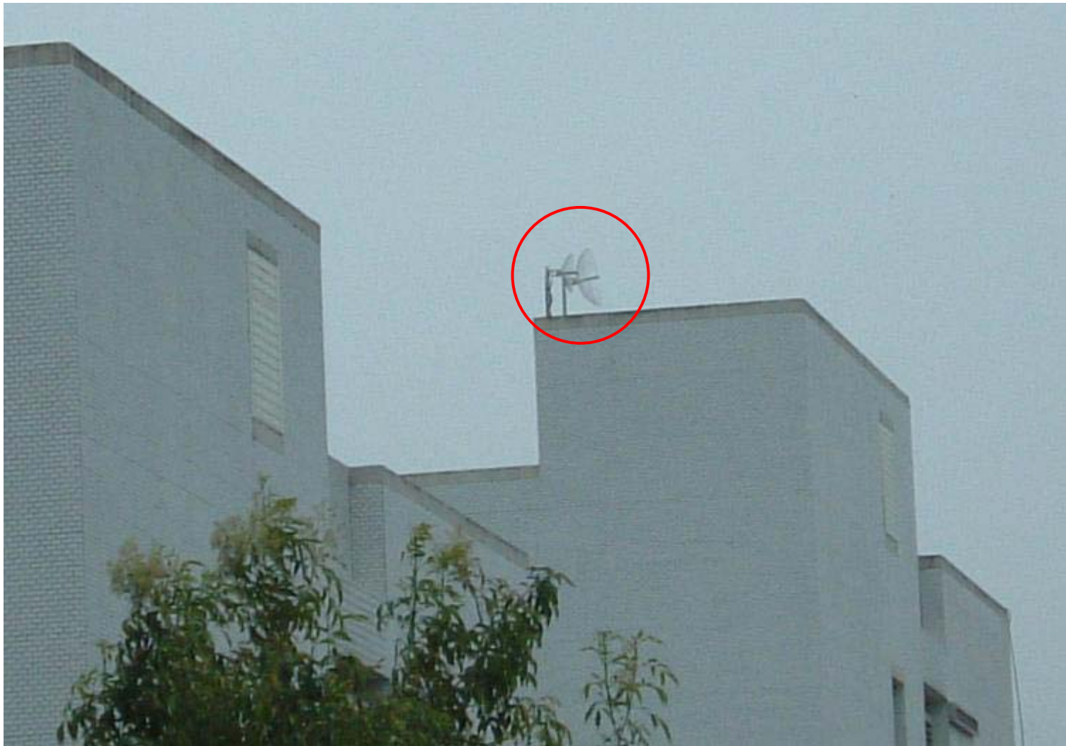
WL-2410 (Slave) with PG-2424 antenna on roof of Inspection Center
