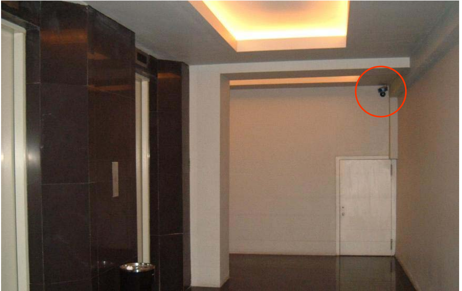
Wireless connected IP camera at lift corner
